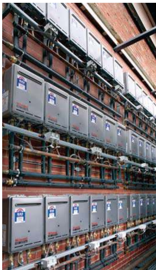
Compact installation of 6 x Manifold Pack 6 External
