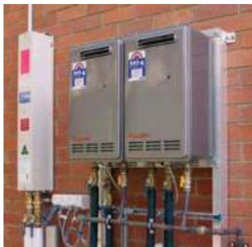
Manifold Pack 2 External Warm Water System with UV Sterilisation
