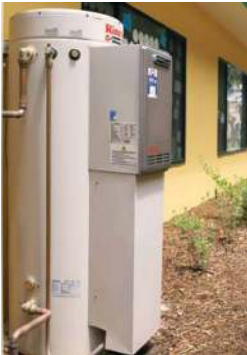
DD1 200 External installed in a narrow side alleyway
