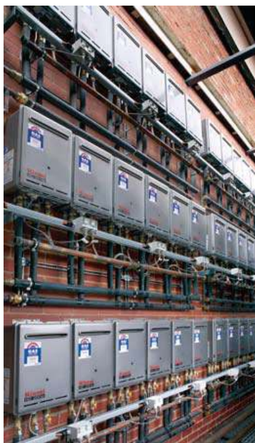
Compact installation of 6 x Manifold Pack 6 External
