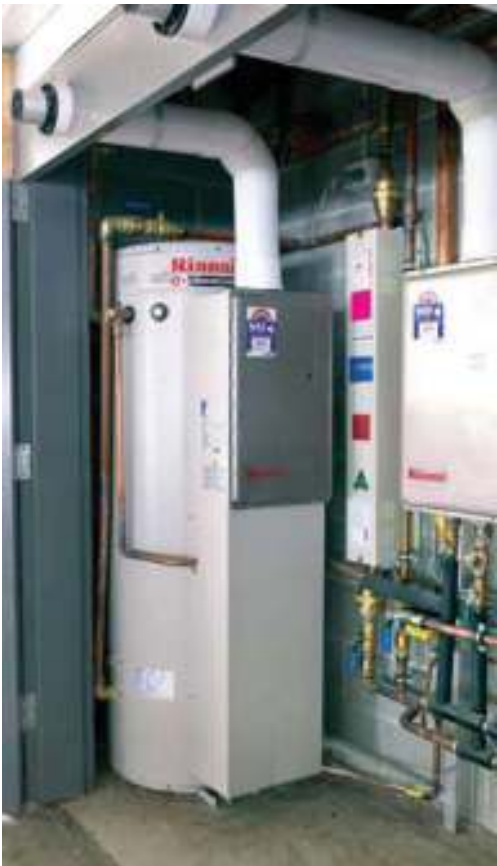
DD1 200 Internal installed in a cupboard
